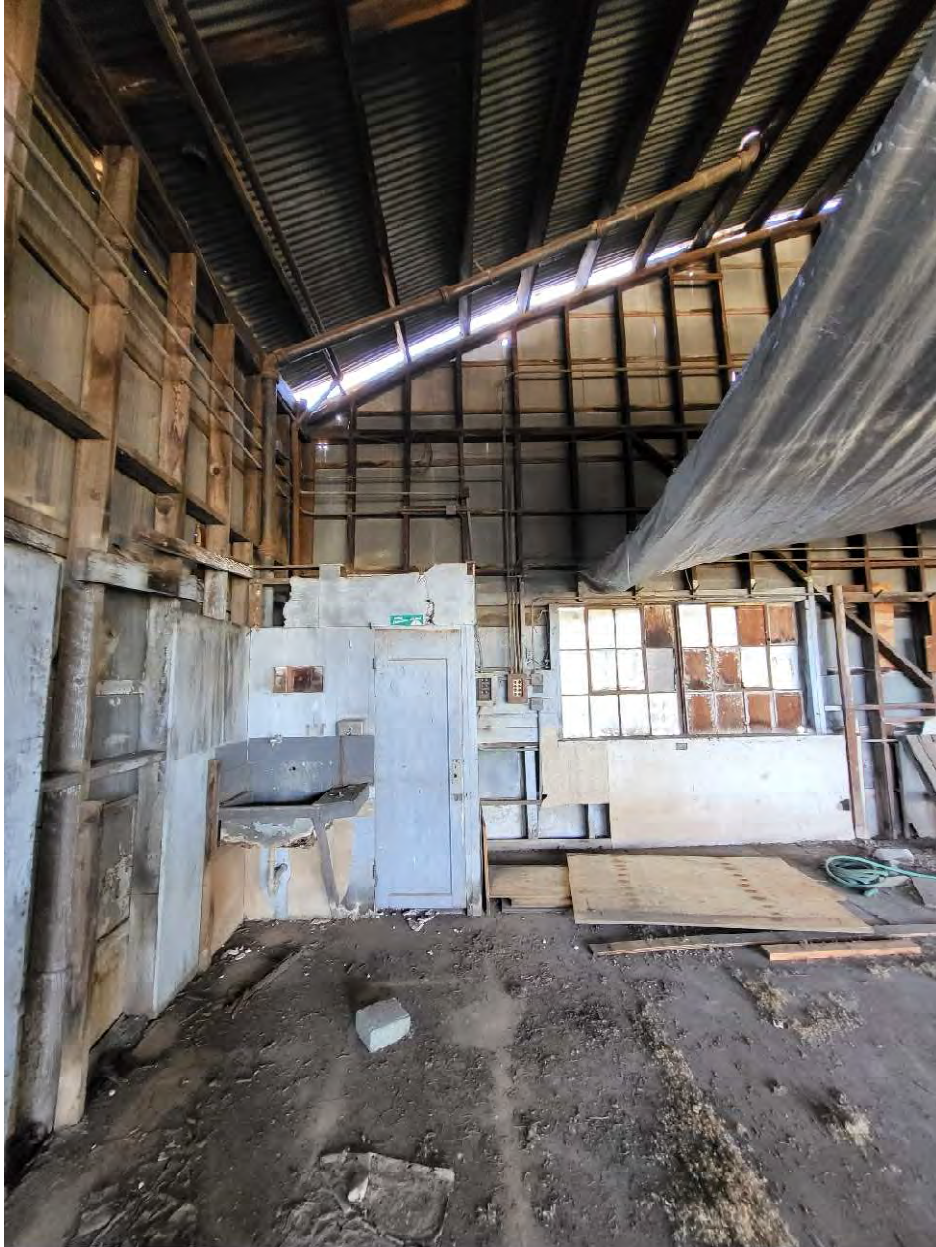
BUILDING 248 – ROOF CONNECTION DISPLACEMENT
